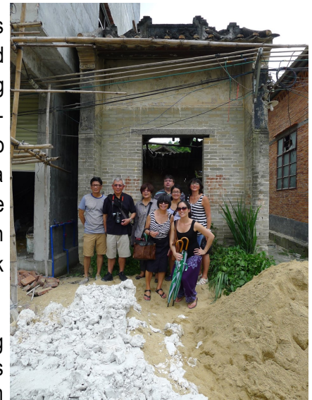
The crumbling Chang's ancestral home
